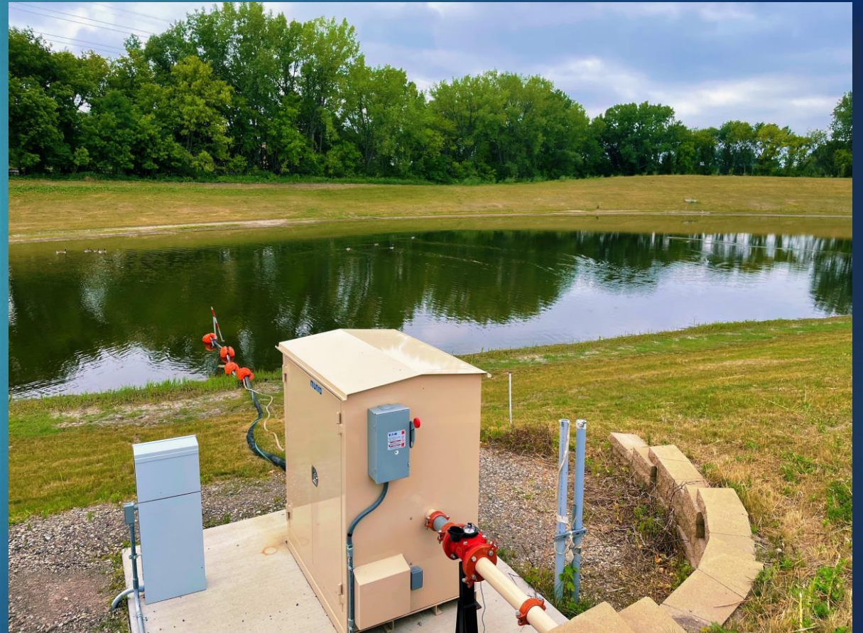
Regional pond and stormwater reuse system
