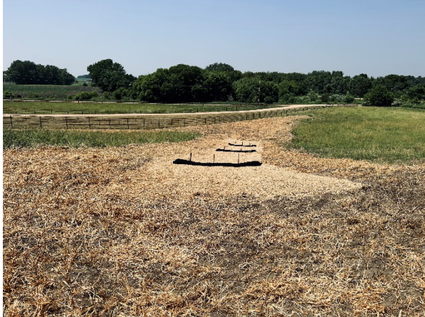
Construction of a grassed waterway in Waconia Township through the SWCD State Cost-share Program.
